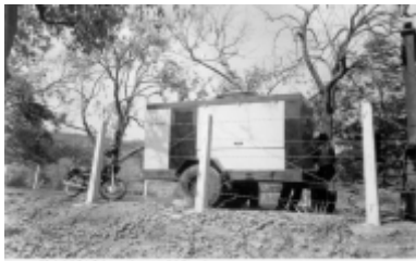
Elgi DPSAC in action at BPCL site
